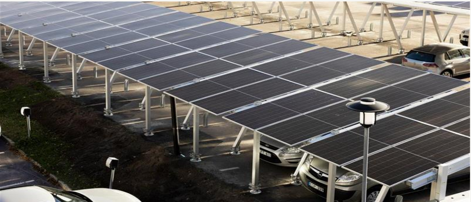
Carports with solar panels at Scandic Luleå
