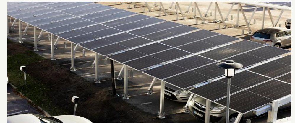
Carporter with solar panels at Scandic Luleå
